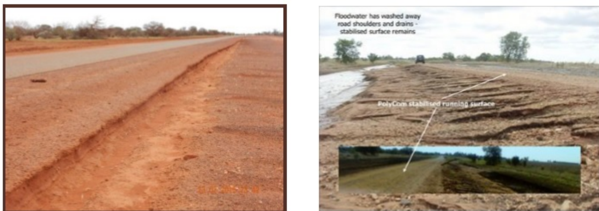
Figure 2: PolyCom Treatment in (L) Western Australia and (R) Queensland, Australia protecting sealed pavement from damage during flood events.
